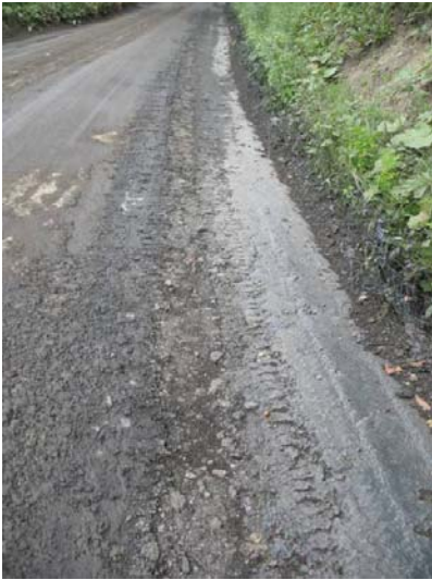
Downhill view, recent E5 application
